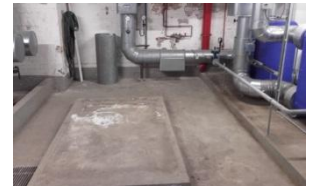
BHKW Campus Ost & Nord
