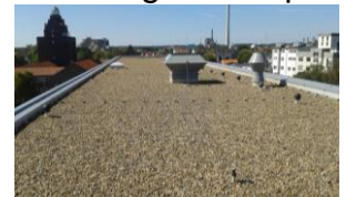
PV Anlagen Campus Ost
